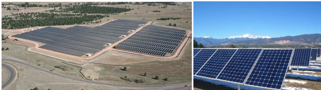
Figure 2-4: The USAFA 5.25 MW solar project
