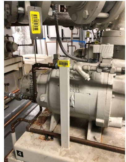
Old water-cooled pump
