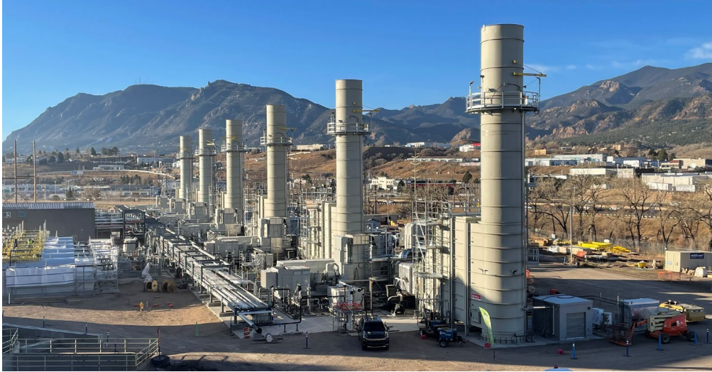
Natural Gas Generators
