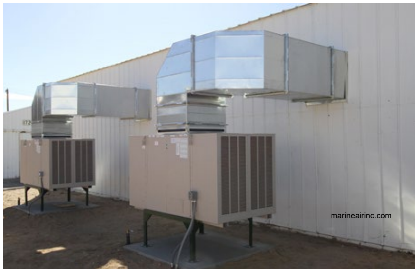
Evaporative cooling in lieu of air conditioning
