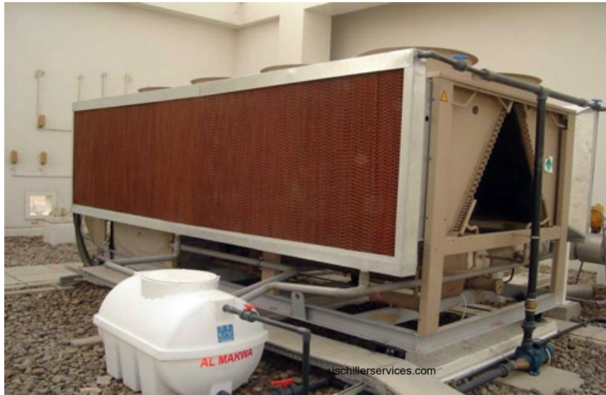
Evaporative pre-cooling pads added to an air-cooled condenser
