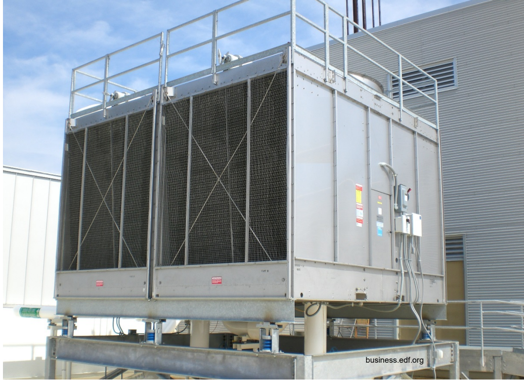
Cooling tower, rejecting heat from water-cooled condensers
