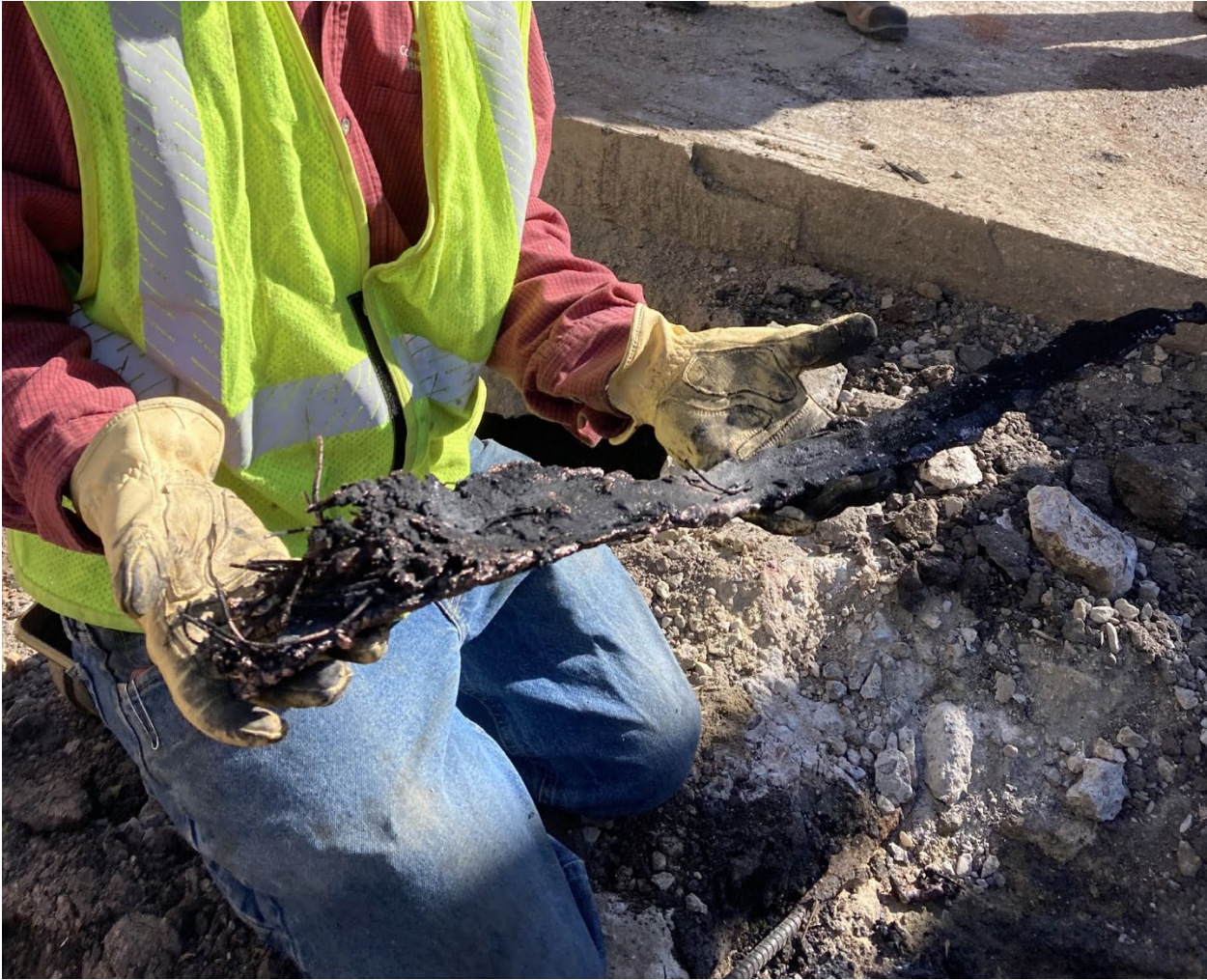
Photo 3 – Damaged cable underneath plywood patch
