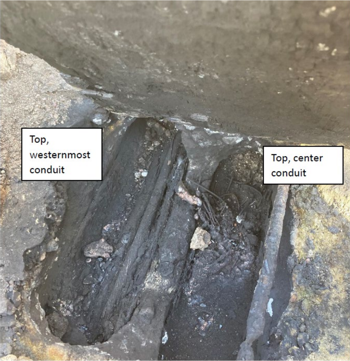
Photo 2 – Damage underneath plywood patch
